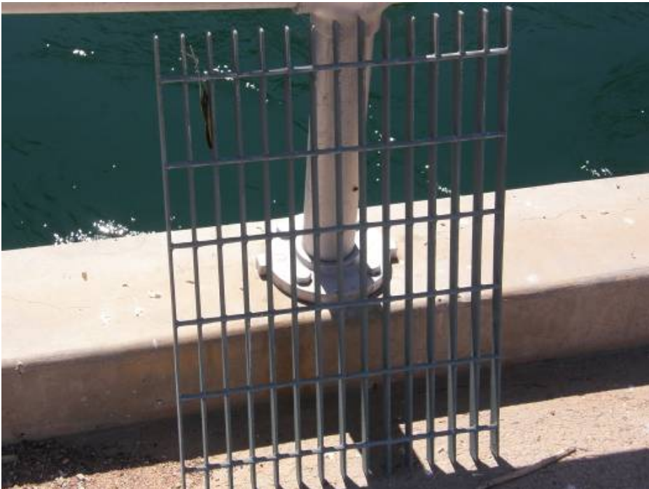
Figure 3.—Coated floor grate before being hung from the forebay trashrack structure at Parker Dam.
