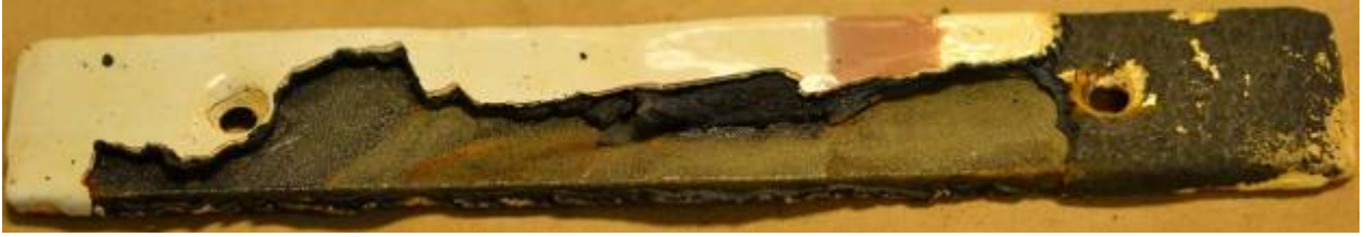
Figure 23.—Failure of overcoated coal tar during a high flow test.
